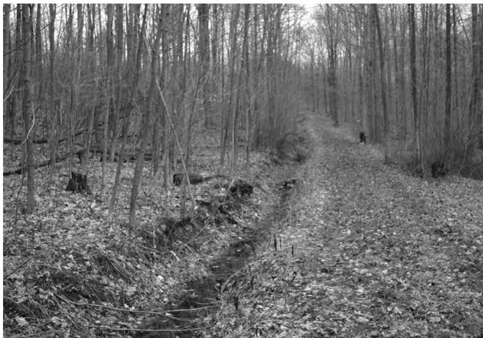
Figure 8. This owner invested in a backhoe and operator to ditch the upslope side of a woods road and pile the spoils onto the road. The result is a nearly year-round road that has served the owners for many years.
