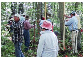
Volunteers dug holes for the wooden posts used on half of the structure.
