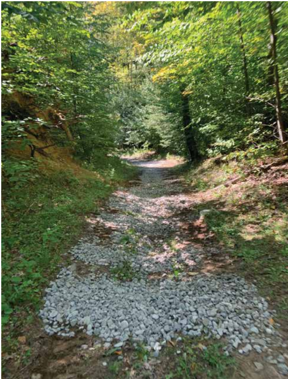
Crushed stone set down as temporary water bars to mitigate damage when accessing the property and to fill in the swale produced from previous erosion of the hill.
