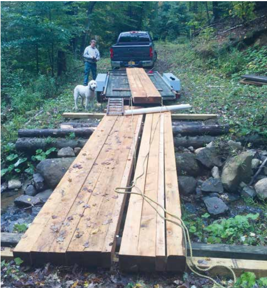
Bruce and Ted planning out the next move to set up a new section of the mini skidder pad for a bridge over the creek. Before this all the equipment to work on the forest was carried up the hill in a pack basket.
