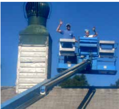
Maureen operating the contractor's lift to paint the cupolas of the barn as part of the farm house and barn renovation project.
