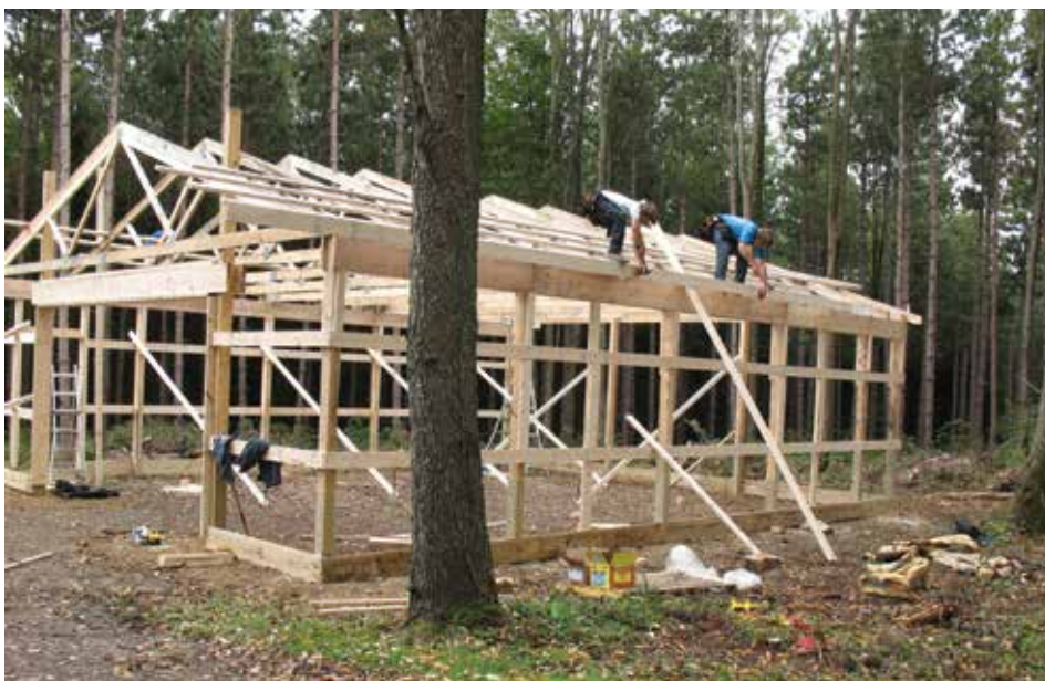
Construction of a pole barn for equipment storage on the DeLellis property.
