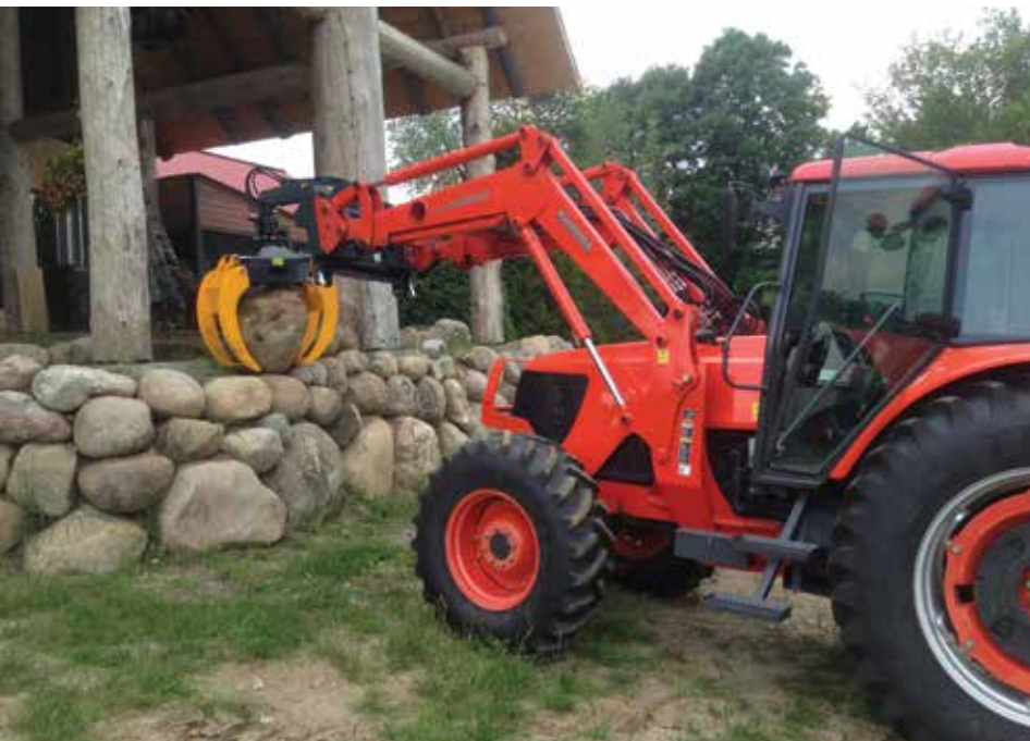
Shown here is a Scorpion grapple, one of the many products offered at Hud-Son Forest Equipment. It was a great asset while building the stone wall shown.
