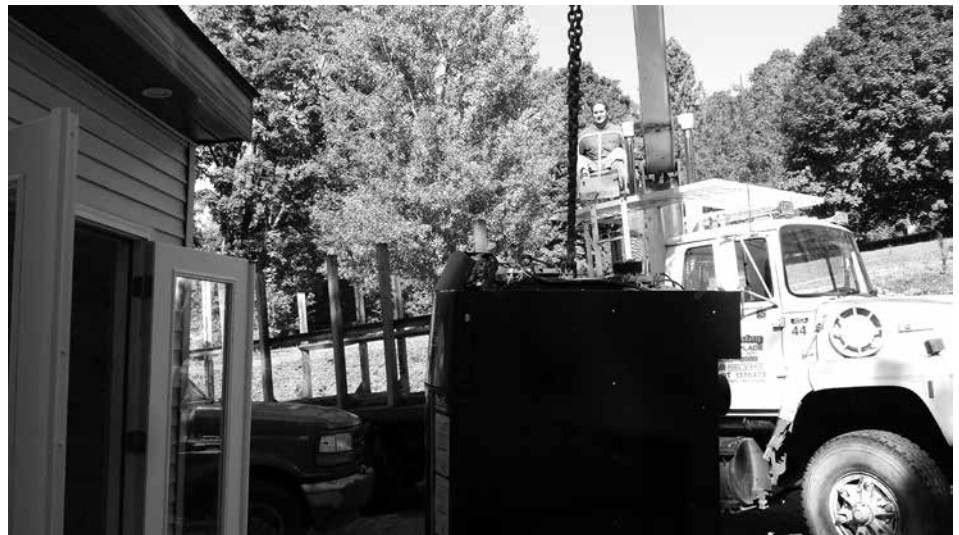
Log Truck setting Flex Fuel boiler into the Shed
