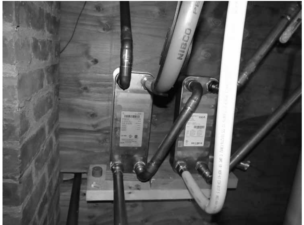
Two Heat Exchangers, 1 for the boiler and 1 for the hot water.
