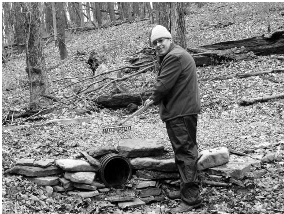
Mark Lewis, MFO, putting the finishing touches on a forest road culvert.
