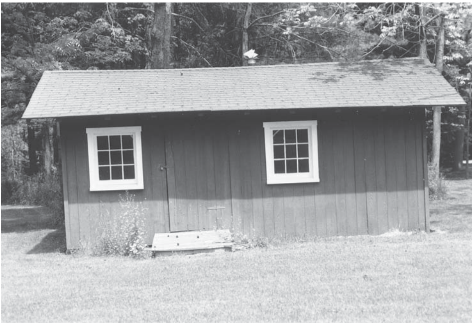
Figure 3. Carpenter bees have heavily infested several boards beneath the overhang of this south-facing outbuilding. This building has only one coat of poorly applied wood stain.
