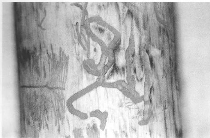
Figure 5. Frass-filled tunnels of a flatheaded borer.
