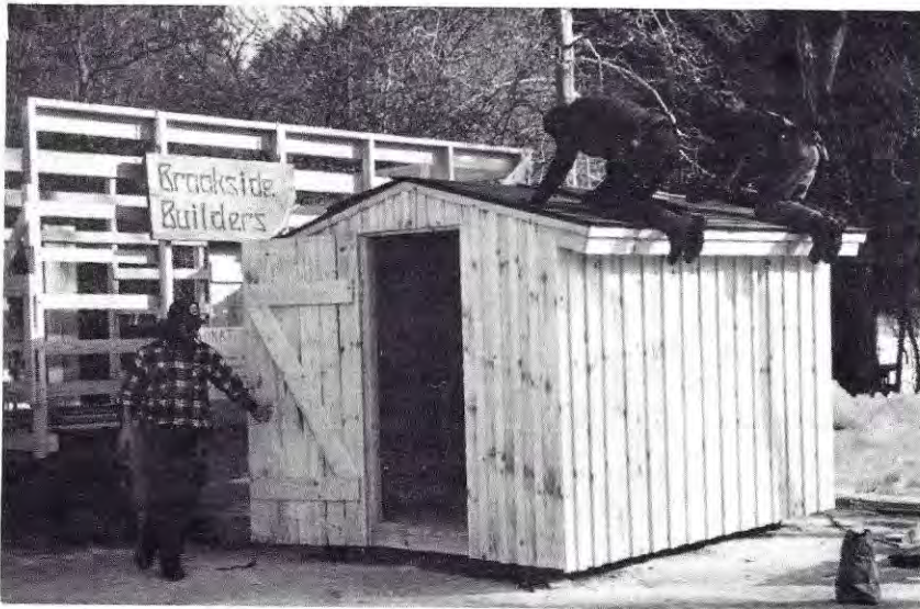
A construction from raw logs done on site for the benefit of 2-3 thousand attendees at the 2-day festival.
