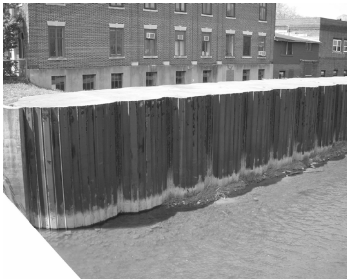
Flood Control Walls on the Allegheny River in Salamanca
